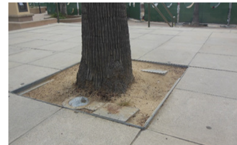
West entry plaza tree well; hazardous surface feature along path of travel.
