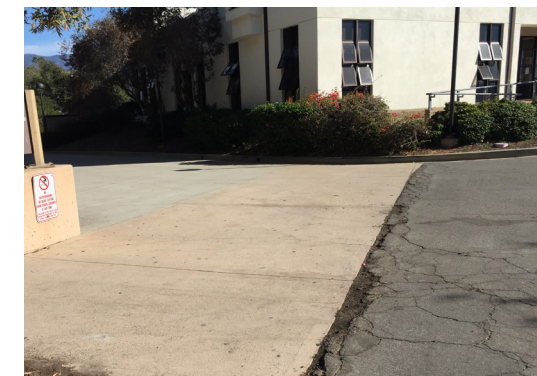
alligator cracking and deterioration at paving transition
