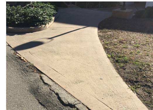
uneven surface and cracking at paving transition from asphalt to concrete
