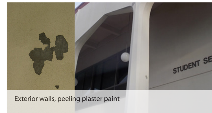
Damaged plaster and paint at corner
