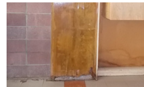
Auditorium walls; water damaged exposed CMU and wood finishes
