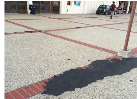
concrete with exposed aggregate and brick accents, patching
