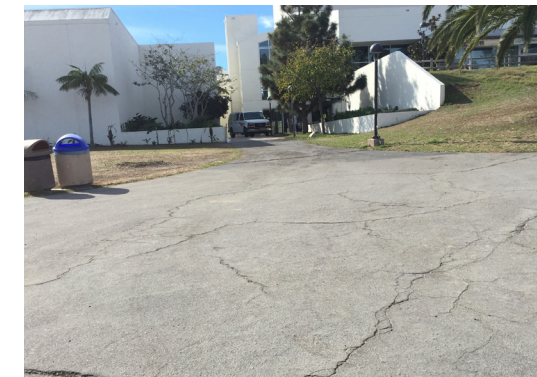
asphalt block cracking
