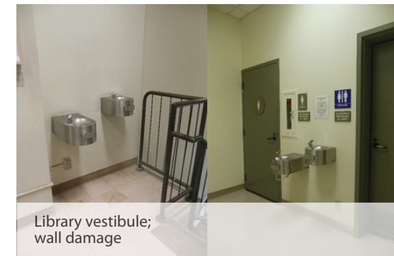
Dispenser and disposal units protrude into required clear space
