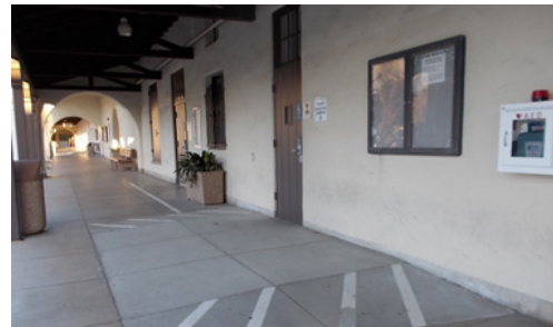
Path of travel interrupted by ramp
