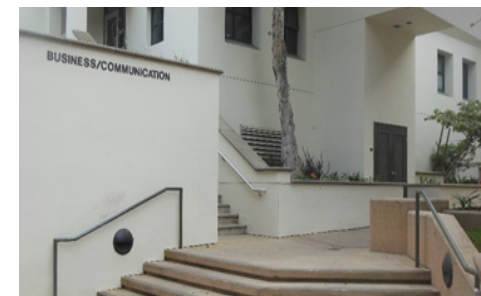
Non-accessible entry lacks wayfinding signs directing user to ramped entry location
