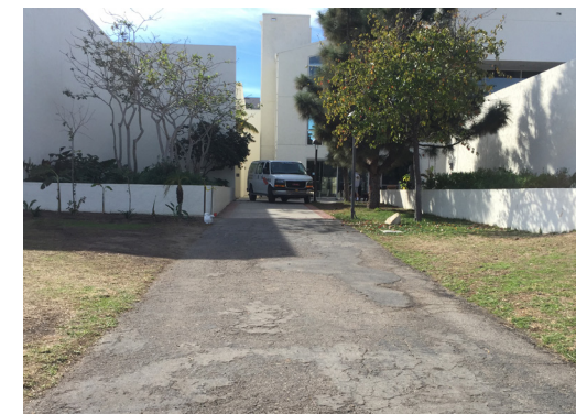
asphalt cracking and surface deterioration
